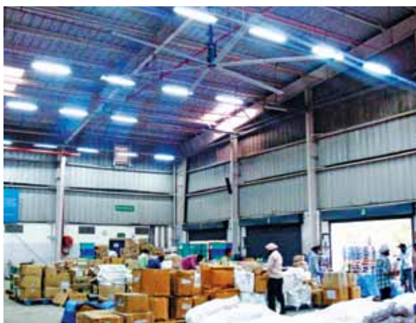
One Kelley HVLS Fan of 24 ft diameter working at a warehouse in Punjab.
